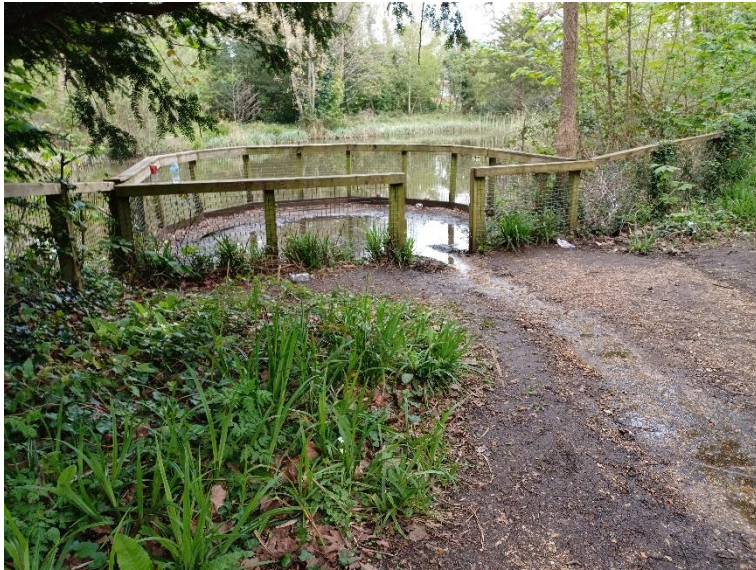
(Above) Flooding of decking/pond-dipping platform caused by drainage failure.
